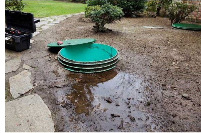
leaking septic system
