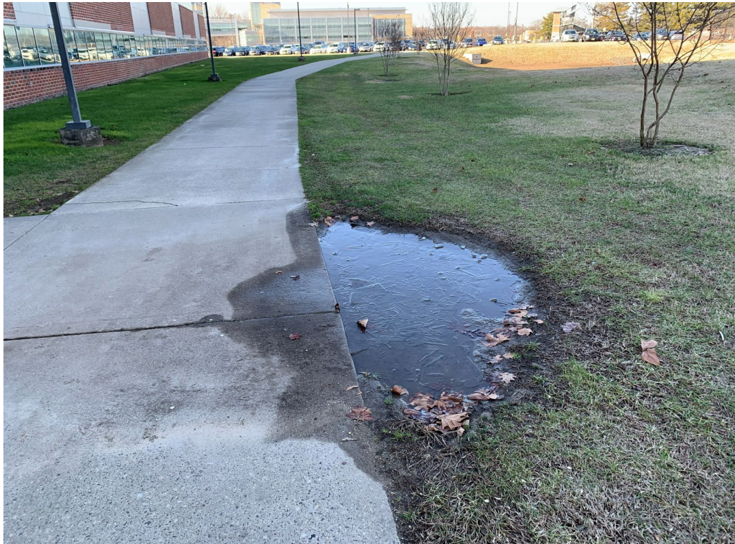
Ponding north of James Hall
