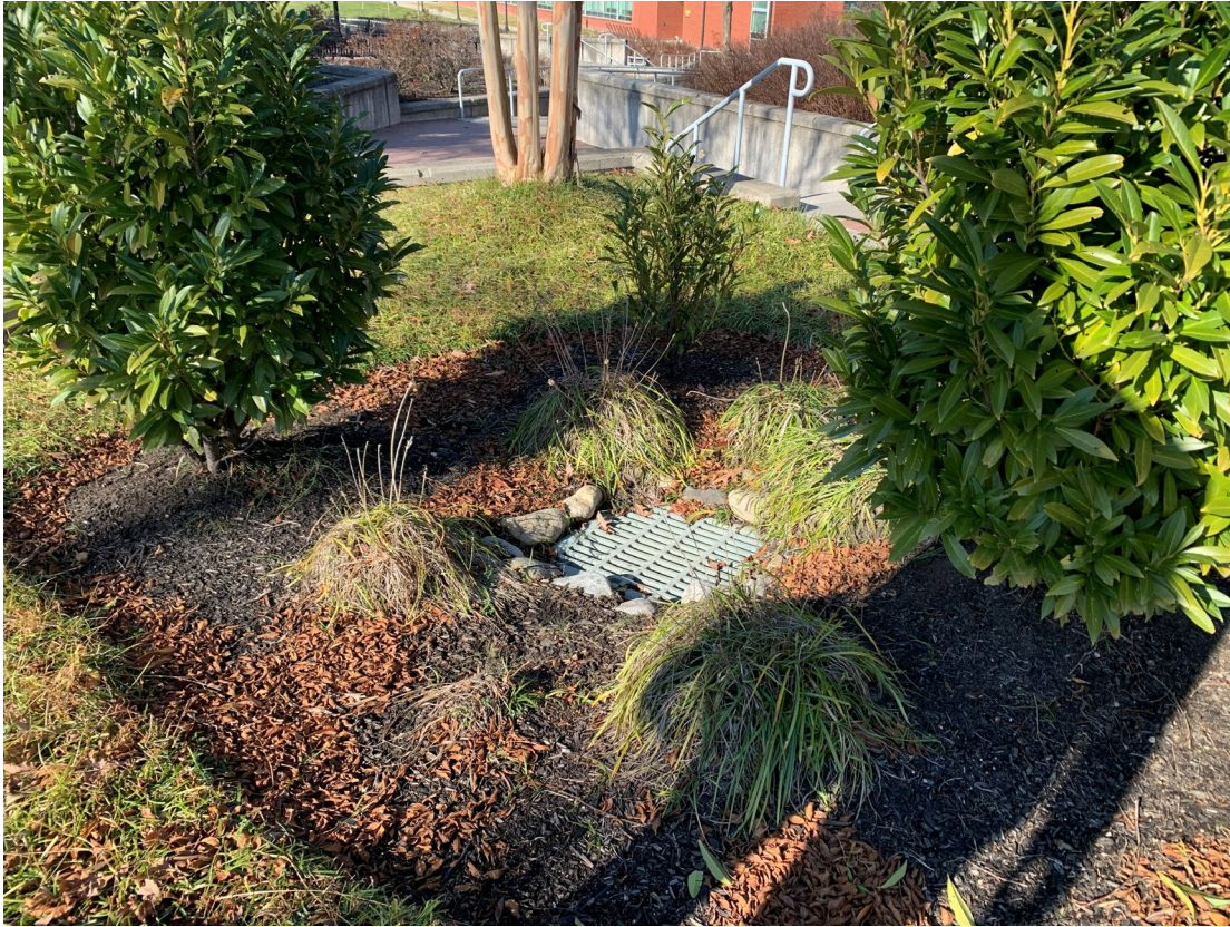
Area inlet in depressed planting bed
