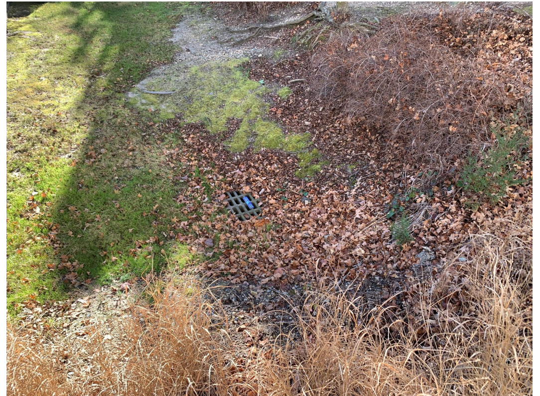
Obstructed area inlet in lawn
