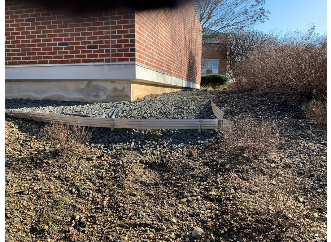
Erosion near Admissions building
