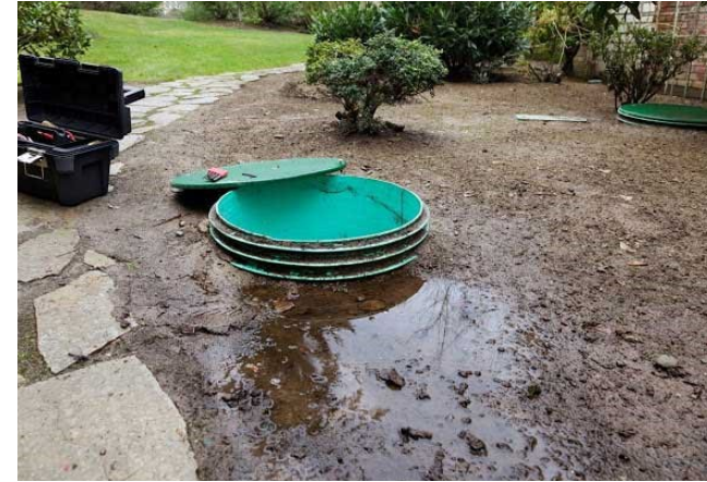
leaking septic system
